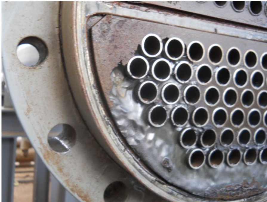
Corrosion of carbon steel tube sheet placed in wet CO 2 , water condensing service.
